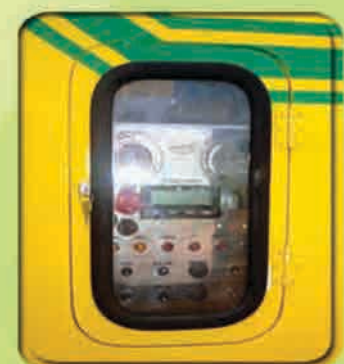
Operation device and main control panel
